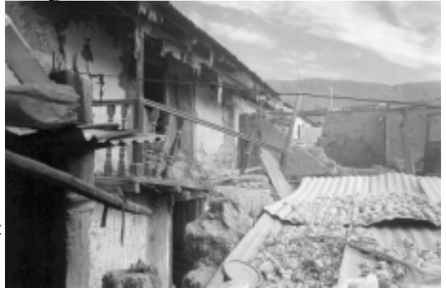
Earthquake damage, Chuquibamba
